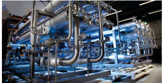
Ultra filtration plant of 30,000 LPH with ozone disinfection, Aquasafe Ethiopia
