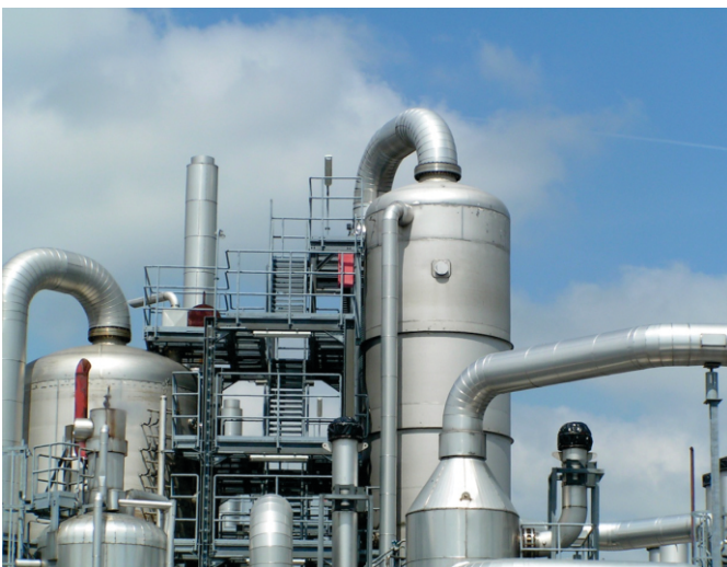
600 TPD solvent extraction plant and meals bagging section
