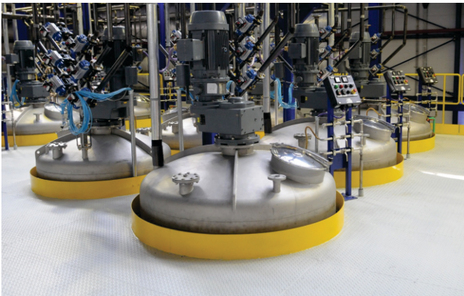
400 TPD Edible oil refinery with soap splitting plant.
